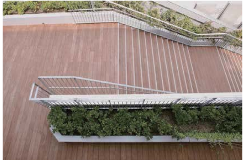
Stairway of an elementary school which Maxelum is applied. Its moderate softness reduces the impact and prevents accidents when children jump or fall down.
